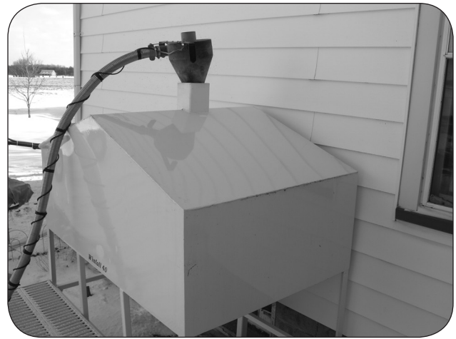
Figure 11. This large welded corn hopper stores about a month's fuel outside a farmhouse. Corn is carried by gravity inside a pipe that passes through a basement window. Inside, the corn flows directly into the stove hopper. The gray hose is used to pneumatically transfer shelled corn from a small wagon to the storage hopper.
