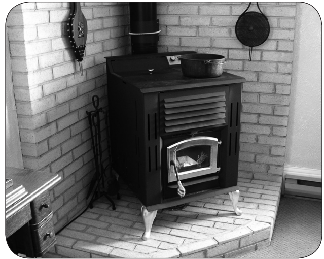
Figure 1. A corn-burning stove sitting in a corner on a brick hearth with ventilated brick on both adjacent walls. The brick creates a non-combustible surface by the stove.
