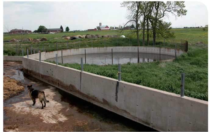
Figure 39. A solid, uncovered outdoor storage with uncovered liquid runoff storage (L1).
