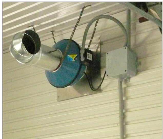
Figure 3. Wall-mounted fan to introduce fresh air into room housing evaporator if activated by pressure switch on the oil burner.
