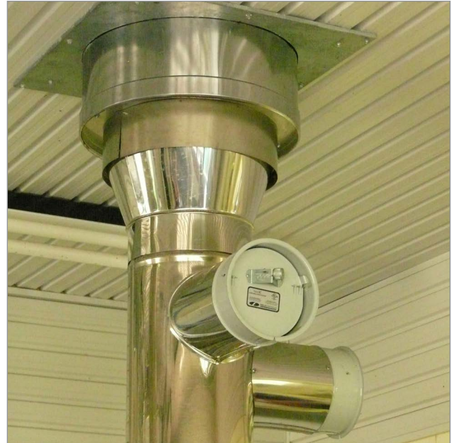
Figure 9. Double-insulated stainless steel smoke stack where stack passes through insulated ceiling/floor or wall.
