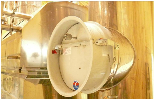
Figure 8. Barometric damper installed on vent pipe.
