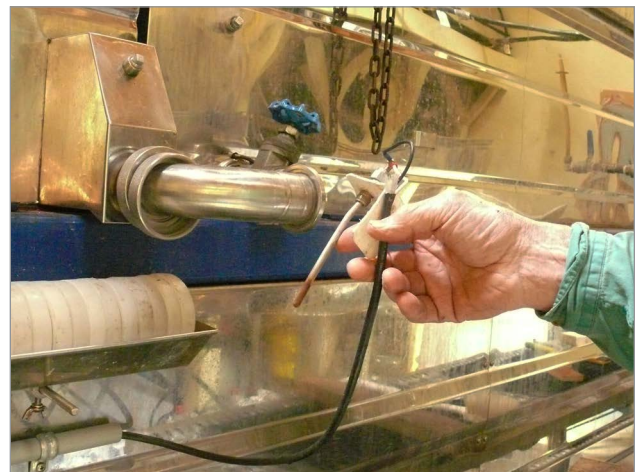
Figure 10. A low-sap level shut-off sensor placed in the float box to the flue pan or into the flue pan directly to measure sap level.
