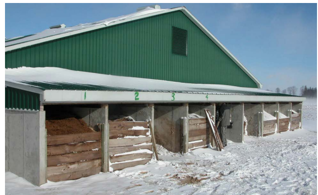
Figure 1. This well-designed bin composter, on a swine farm, was working effectively the January day this photo was taken, when the air temperature was -15^{\circ}\text{C} .
