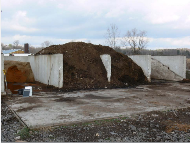
Figure 3. This bin compost system (for swine) has four bins; filling, primary heating, secondary heating and substrate storage. Bins are not normally filled to overflowing. The apron floor area out front encourages clean-up and is sloped away from the bins in all directions. Bin floors are sloped slightly to the back. The operator said he would make the apron area bigger if doing it again.
