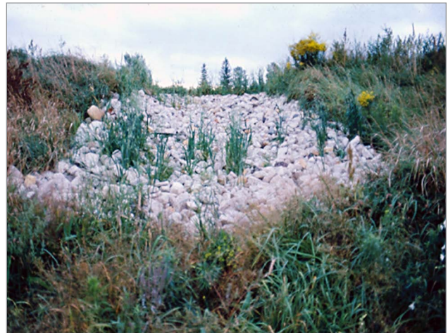
Figure 3. A rock chute spillway located at the outlet of a grassed waterway.
