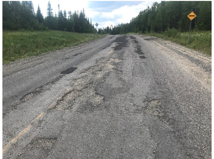
An example of road surface pavement damage.
