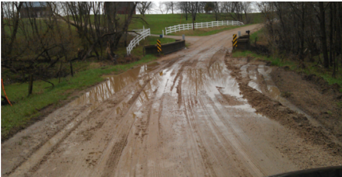
Rutting and surface damage shown on an unpaved road.
