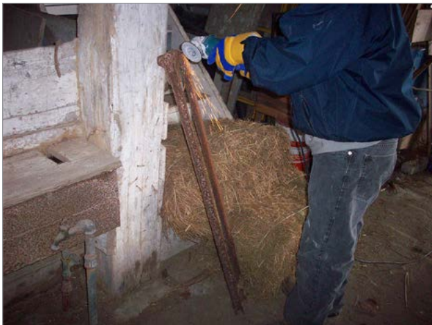
Figure 4. Grinding a piece of steel in close proximity to combustible materials.
