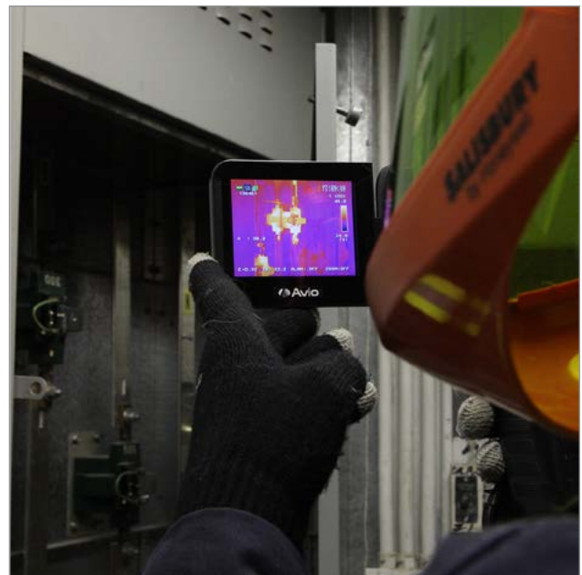
Figure 5. Inspection of electrical equipment by insurance company. Source: Heartland Farm Mutual, Ontario.
