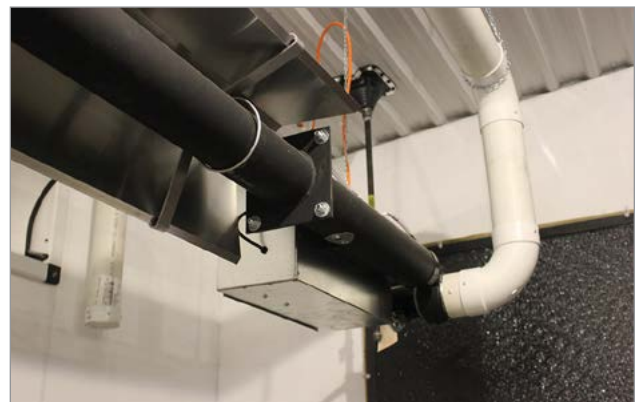
Figure 8. Radiant tube heater suspended in barn.
