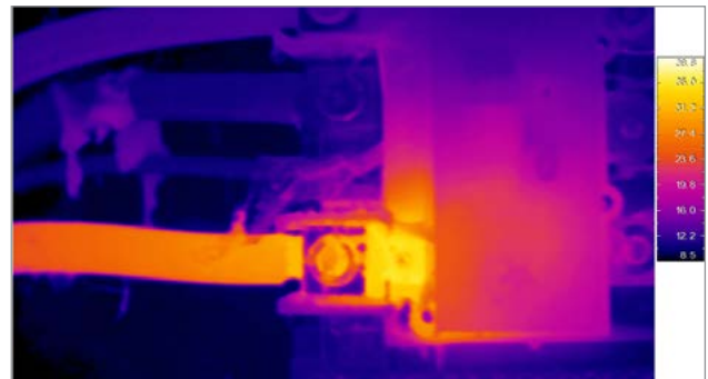
Figure 3. Thermographic picture of an electrical panel. Source: Heartland Farm Mutual, Ontario.
