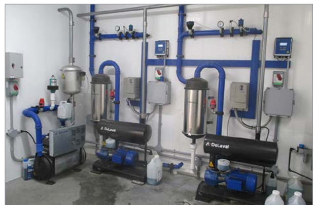
Figure 1. Equipment room free of clutter, dust and debris. Source: Heartland Farm Mutual, Ontario.
