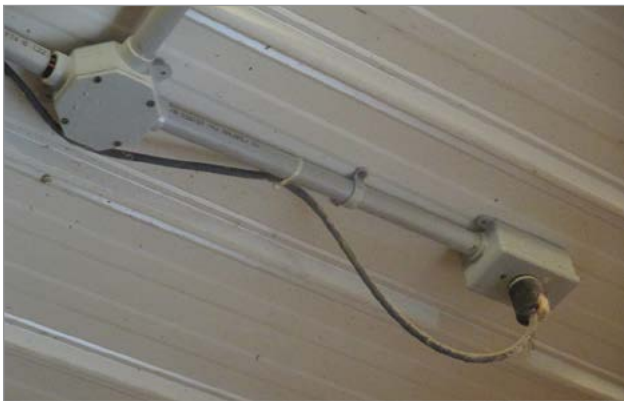
Figure 2. Temporary electrical equipment plugged into receptacle in livestock area. Source: Heartland Farm Mutual, Ontario.
