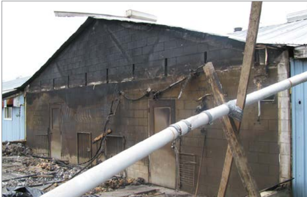
Figure 7. Example of an intact fire separation that did its job and prevented fire from spreading through the barn. Source: R. Drysdale, Farm Mutual Reinsurance Plan.
