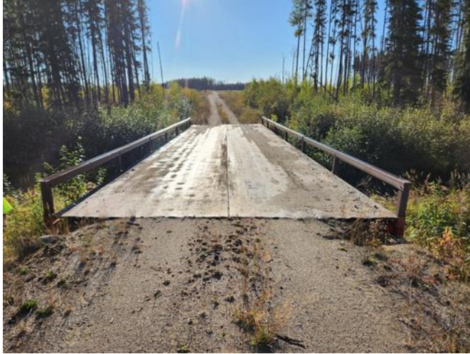
Figure 7. An example of a bridge without proper signage and showing minor erosion.
