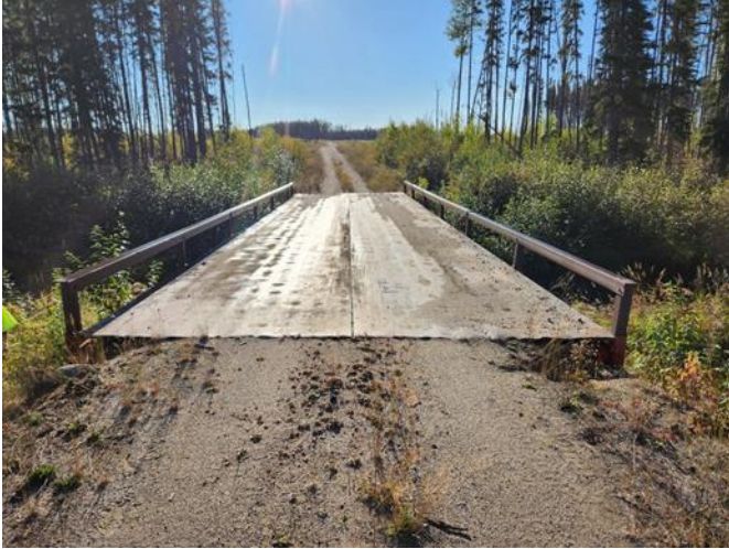
Bridge with no signage and some minor erosion.
