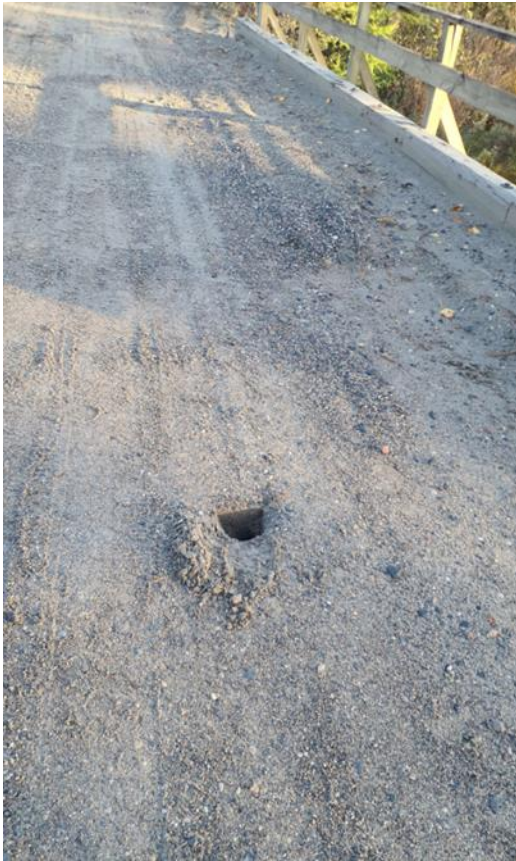
Figure 9. Photo of bridge with gravel on deck on Greta Road.
