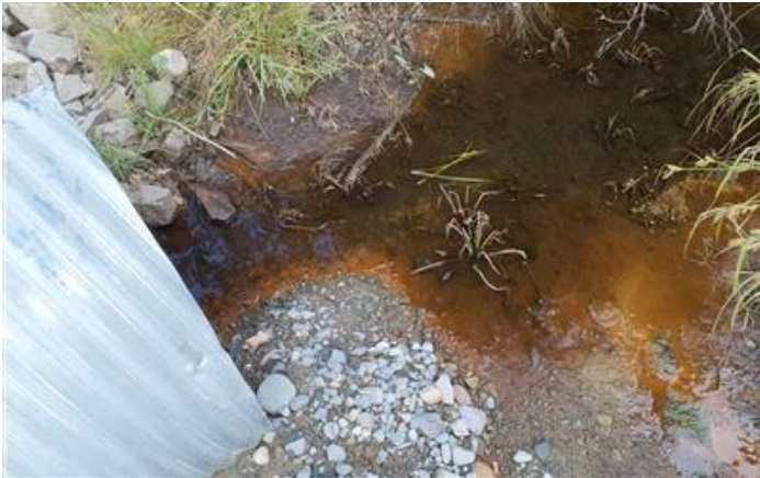
#P11-55 – road building material eroding into watercourse
