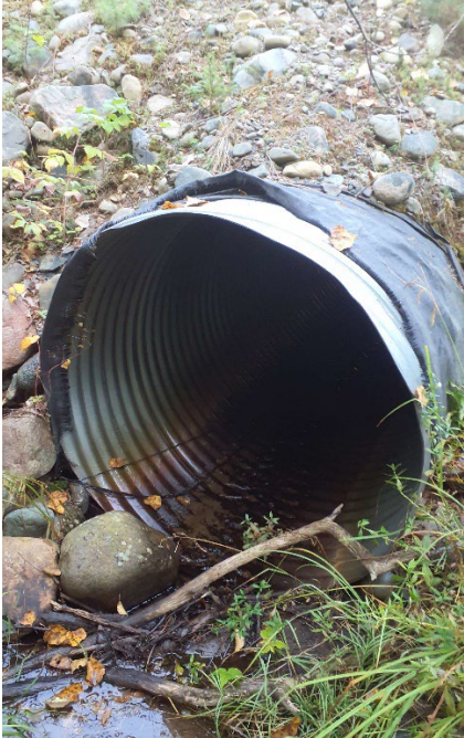
#6782 – perched culvert with rip rap into watercourse
