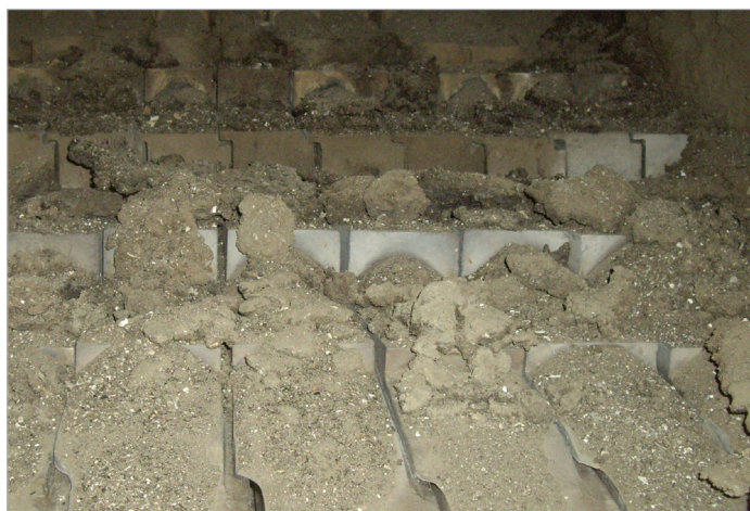
Figure 3. Clinkering results in jamming of furnace elements. Source: CanmetENERGY.
