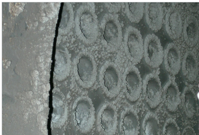
Figure 4. Boiler tube fouling leads to decreased efficiency. Source: CanmetENERGY.
