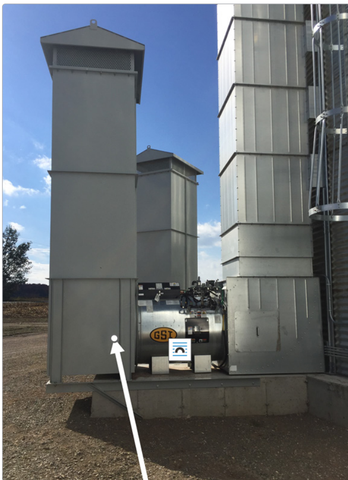
Figure 7. Dryer fan with silencers.
