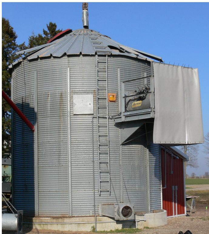
Figure 8. A heavy, flexible, weather and heat-resistant sound blanket panel installed in front of a bin dryer on the side of a grain storage bin.
