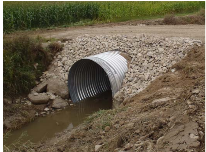
Figure 3–1. A wider crossing recently installed on a drain. Source: Dietrich Engineering Limited, Waterloo, Ontario
